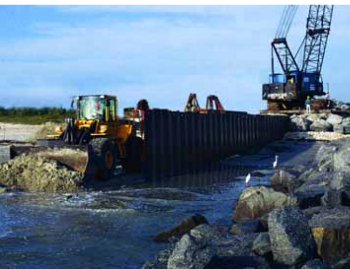
Steel sheet pile being added to the jetty to help reduce the amount of sand that can get into the inlet
