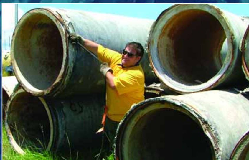
Rubber seals being removed from concrete water pipes prior to placement on the reef site
